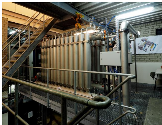
Figure 2. Picture of the ceramic membrane filtration demonstration plant at Vitens production location, Wierden, NL
